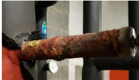
Before repairs with ZINGA
