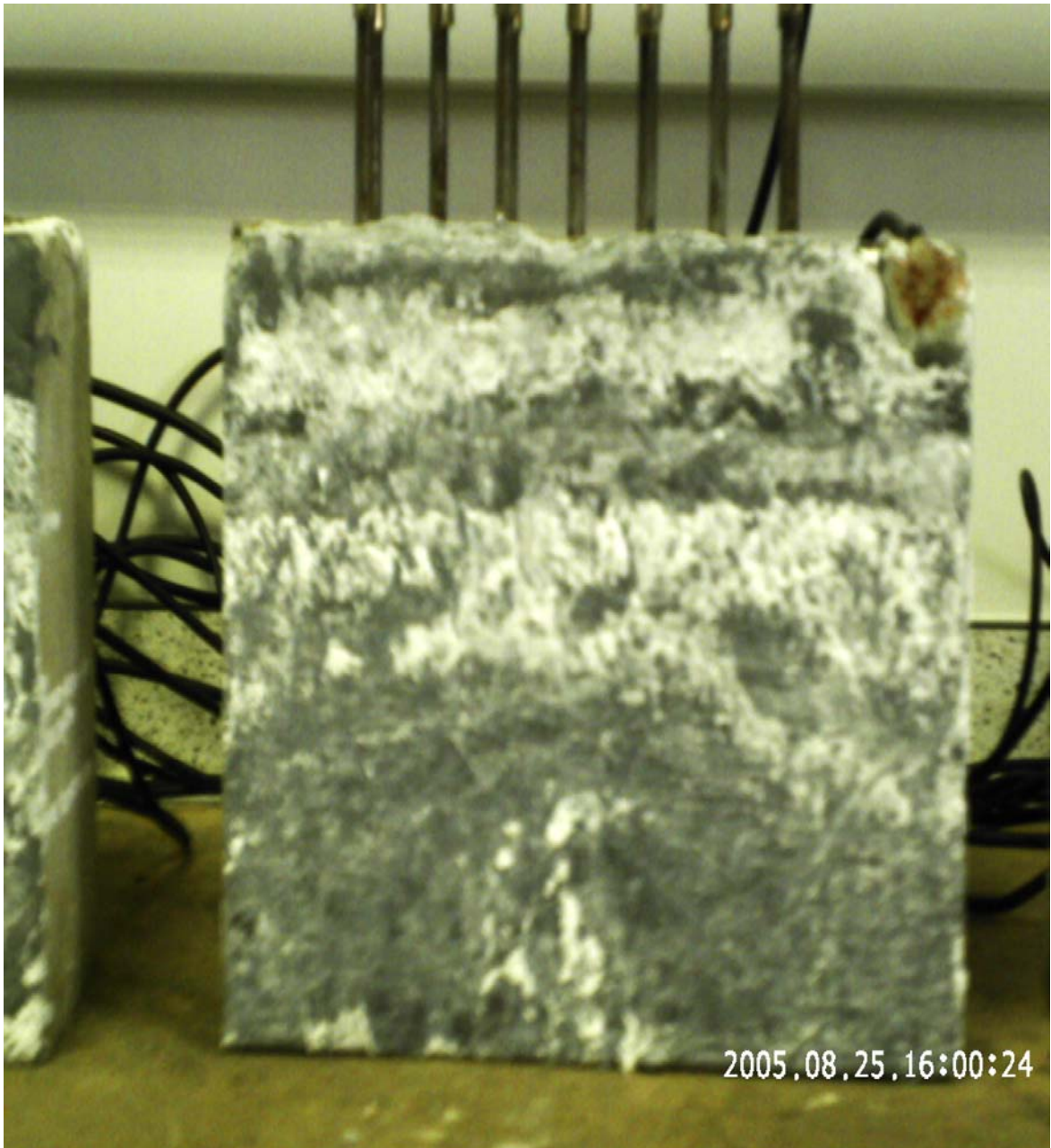
Concrete block one (Zinga without LiCl) with corrosion products masking the surface.
